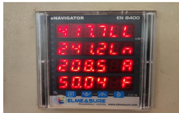
Fig. 5: Digital Energy Meter Readings.
