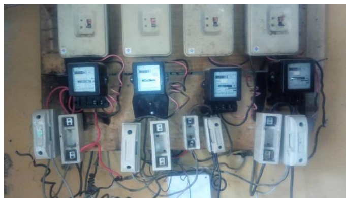
Fig. 2: Electricity Theft by Bypassing the Meter.
