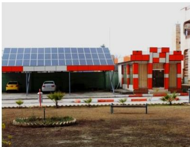
Fig. 6: The Real Practical Structure of the Solar Power Plant (Technical College of Mosul).
