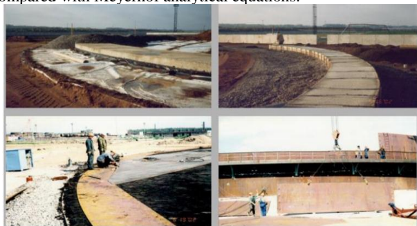
Fig1: Ring Shallow Foundation For Large Storage Tank Designed By Russian Company (Petergib), From Achieve Of The First Author Of This Article.
