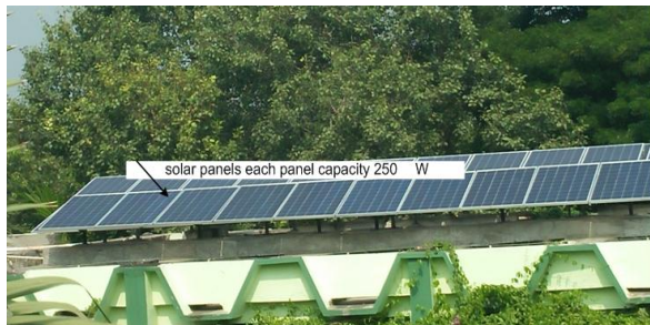
Fig. 16 :Solar Panels connected in series
