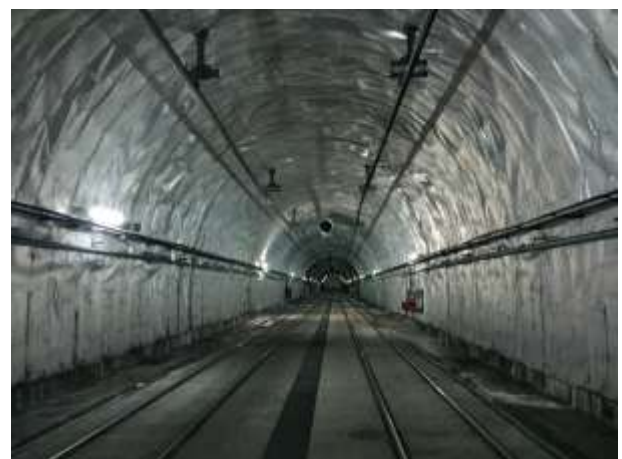
Fig. 1: Image of the tunnel during the data collection phase. The image corresponds to the tunnel on its way through Mount Benacantil.
