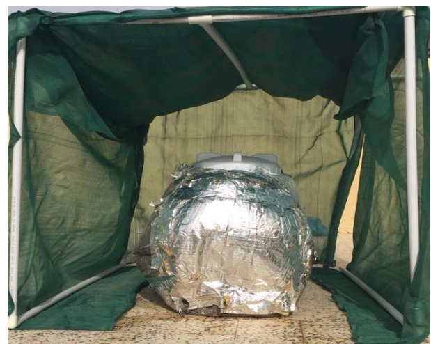
Fig. 3: Overhead Water Storage Tank with Insulation and Shade (Case 4).
