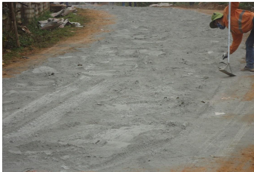
Fig. 1: Cement Placement on the Road before Mixing with Local Clayey Soil Underneath.
