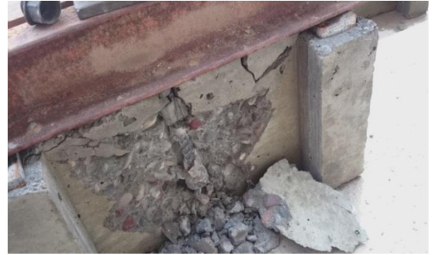
Fig. 10: Explosive Side-Face Blowout.
