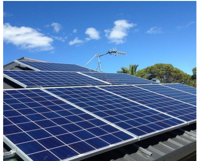
Figure 1. Photovoltaic Electrical Power Generation Site
