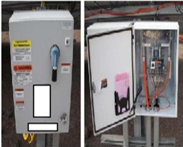
Figure 2. (a) Combiner Figure 2. (b) Tie Box
