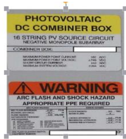
Figure 3. Arc Flash Warning Label on CombinerBox
