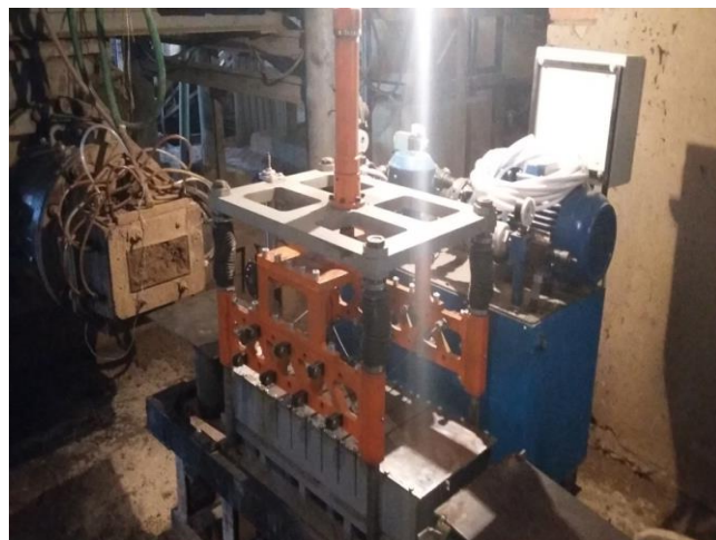
Fig. 11: General view of the modernized technological equipment for the formation of brick during installation work in a real enterprise.
