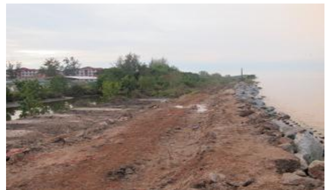
Fig. 6: Eroding shoreline at Sungai Tengi (2016).
