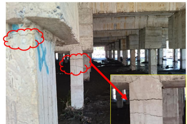
Fig. 7: Crack underneath of pile
