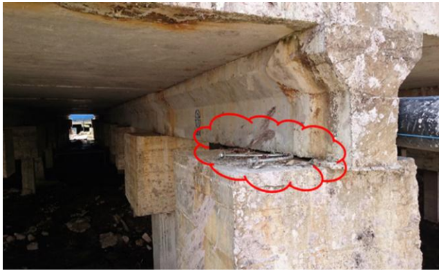
Fig. 4: Gap between pile cap and pre-cast beam
