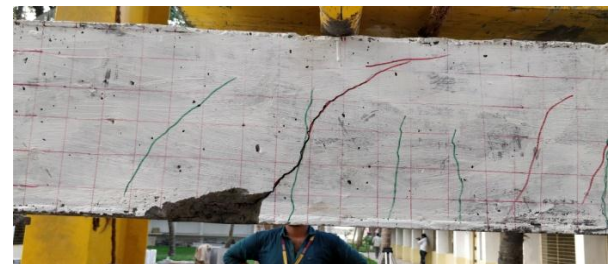
(b) Crushing of concrete in BWSC-2
