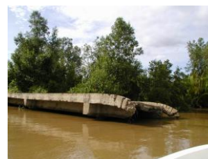
Fig. 1: Remains of collapsed wharf at Sg. Saribas
