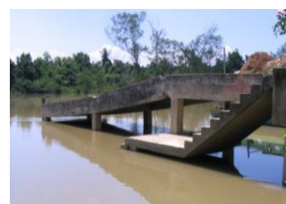
Fig. 3: Failure of a jetty at Kpg. Hulu, Samarahan Division
