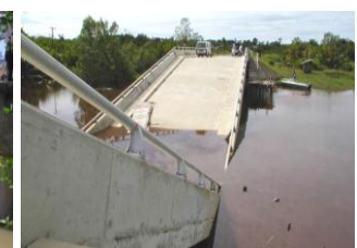
Fig. 4: Collapsed Sg. Palasan Bridge in Betong Division
