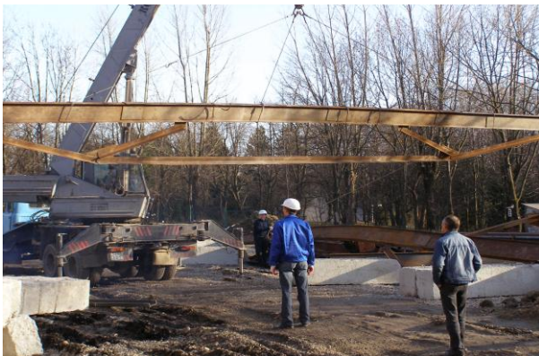
Fig.14. Installing of low element sub diagonal truss with span L=18m, Sanatorium "Zeneva" Truskavets, Ukraine
