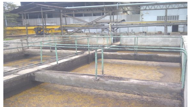
Fig. 3: Condition Before Repair.
