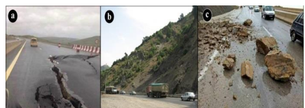
Fig. 1: A) Landslides Affecting A1 Highway; B) Landslides Affecting (RN5) National Road; C) Rockfall on Chiffa-Médéa National Road (RN1).
