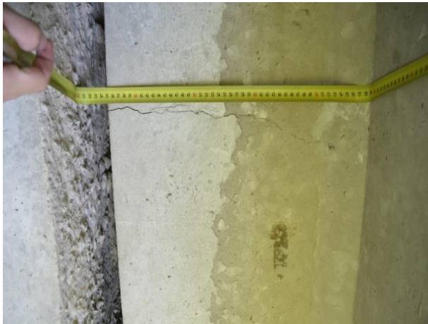
Fig. 4: A Crack in A Reinforced Concrete Structure.
