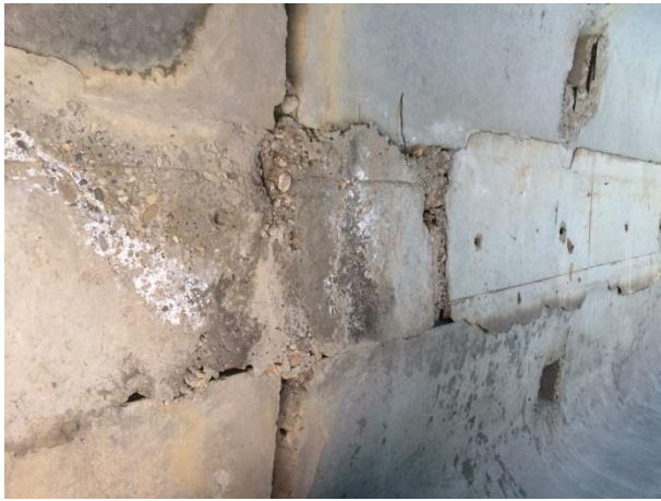
Fig. 3: Corrosion of Reinforced Concrete Elements.
