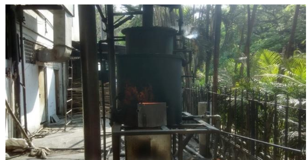
Fig. 1: Wood Ash Burning Boilers.
