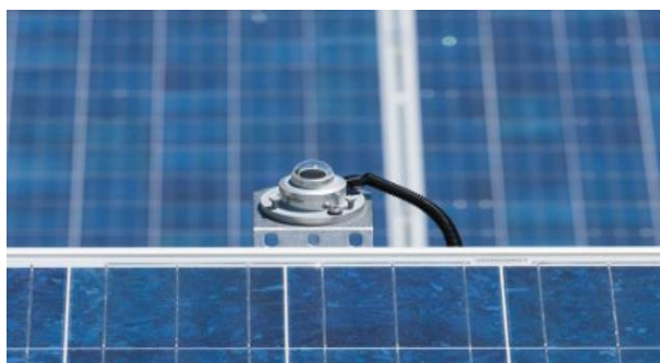
Fig.3: With Sensor to Detect Vibration of Solar Module.
